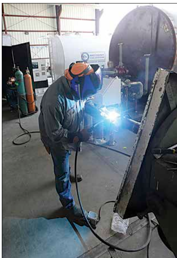
Mike Provencio welds tubing for a fueling station, one of 12, for a customer in Alabama.
