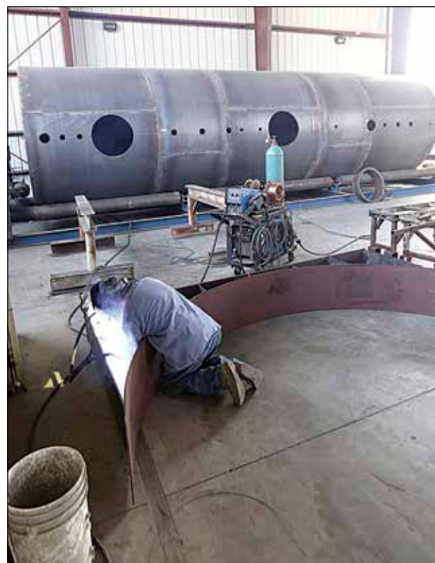
A welder works on a saddle for a 20,000-gallon tank for a local customer.
