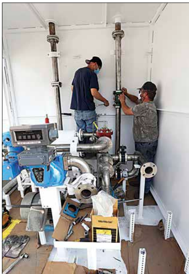
Inside one of 12 fueling stations being manufactured by Bryant Fuel Systems, Dillon Allen, left, and Toby McCaslin work on final assembly for delivery to Alabama.
